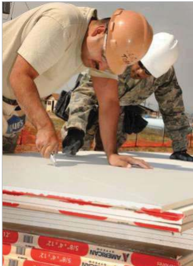
Senior Master Sgt. Angel Torres and Tech. Sgt. Rodney Allen, 113th Civil Engineer Squadron structuralists, cut sheet rock for a humanitarian rebuilding effort at Window Rock, Ariz., June 1, 2011. The 113th CES members are in Window Rock as part of the Innovative Readiness Training, a civil-military affairs program linking military units with civilian communities for humanitarian projects. (U.S. Air Force Photo by Tech Sgt. Craig Clapper)
