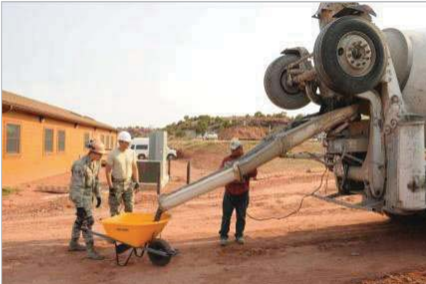
Members of the 113 CES collect cement during a humanitarian rebuilding effort in Window Rock, Ariz., June 1, 2011. The 113 CES members are in Window Rock as part of the Innovative Readiness Training, a civil-military affairs program linking military units with civilian communities for humanitarian projects. (U.S. Air Force Photo by Tech Sgt. Craig Clapper)
